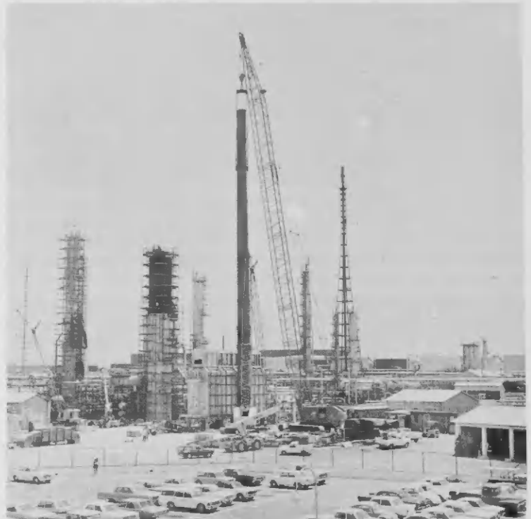
The L2AR's 150-ft stack is back in place against its furnace following refractory lining to its interior.
